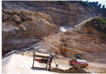
Simultaneous operation of left plinth formwork, preparation of dowel execution, compaction of body rock fill layer and instrumentation cable protection
