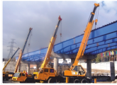
Installation of metal decks of the bridge in two shifts due to heavy traffic
